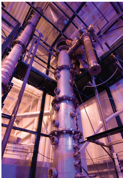
SRI designed this reactor, which uses a proprietary carbon sorbent to remove CO 2 from flue gas.
