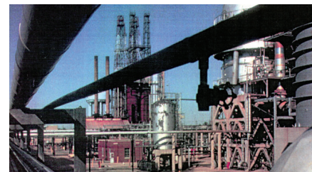
Aging pipes and vessels in an oil refinery
